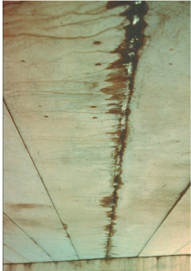
Figure 7.7.4 Leaking Joint between Adjacent Slab Units
