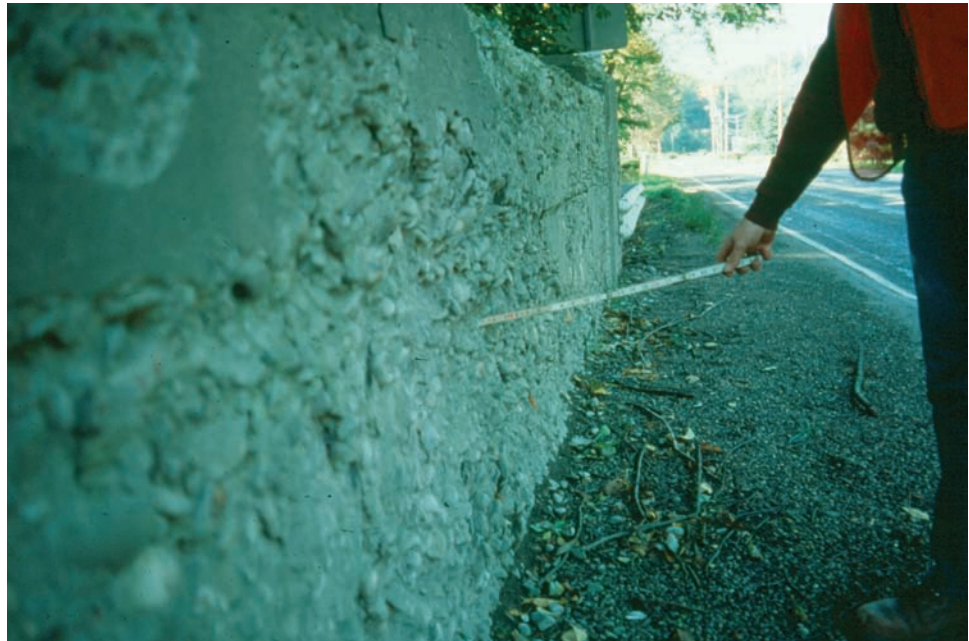
Figure 7.3.9 Close-up of an Interior Face of a Through Girder with Heavy Scaling due to Deicing Agents
