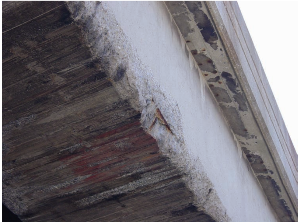
Figure 7.2.20 Collision Damage to Tee Beam Bridge Over a Highway
