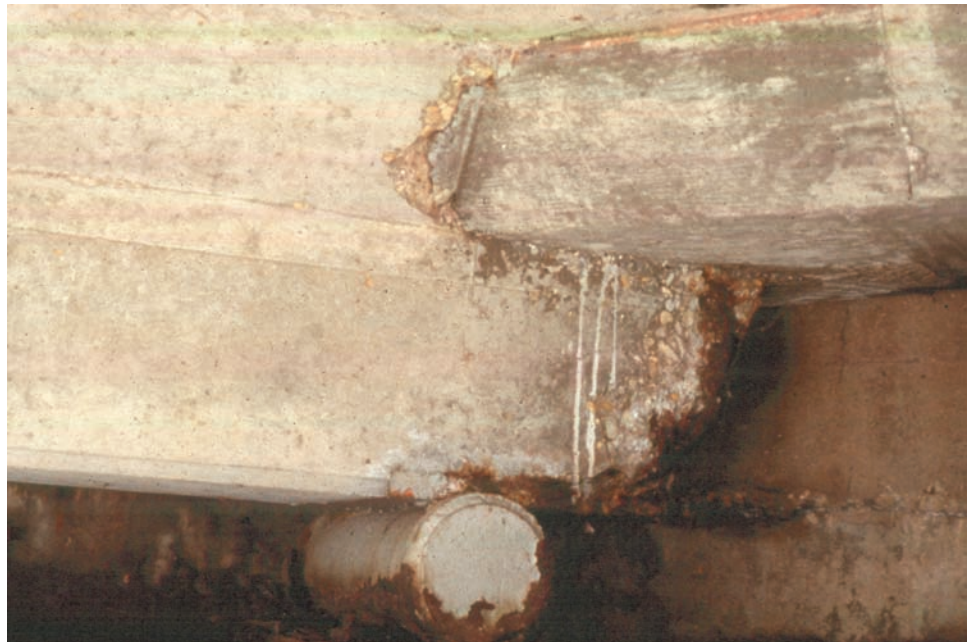
Figure 7.2.9 Spalled Tee Beam End
