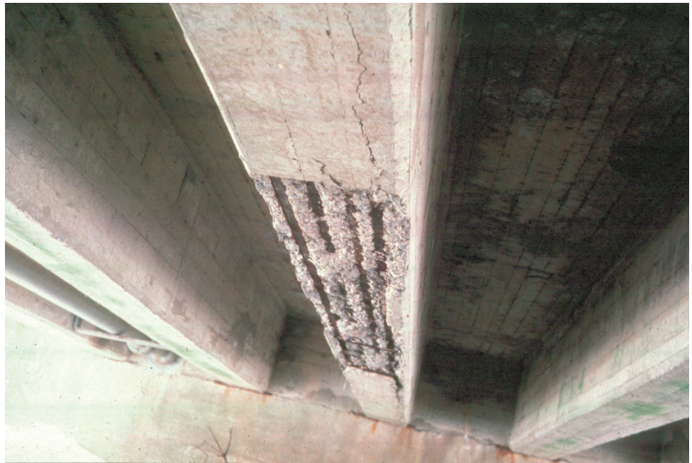
Figure 7.2.16 Spall on the Bottom of the Stem of a Cast-in-Place Tee Beam with Corroded Main Steel Exposed
