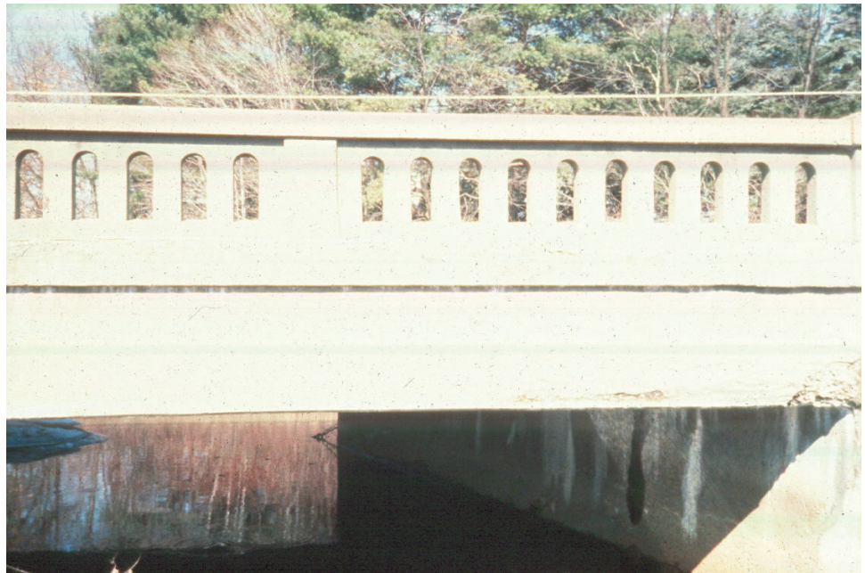
Figure 7.2.19 Deteriorated Tee Beam End Due to Drainage
