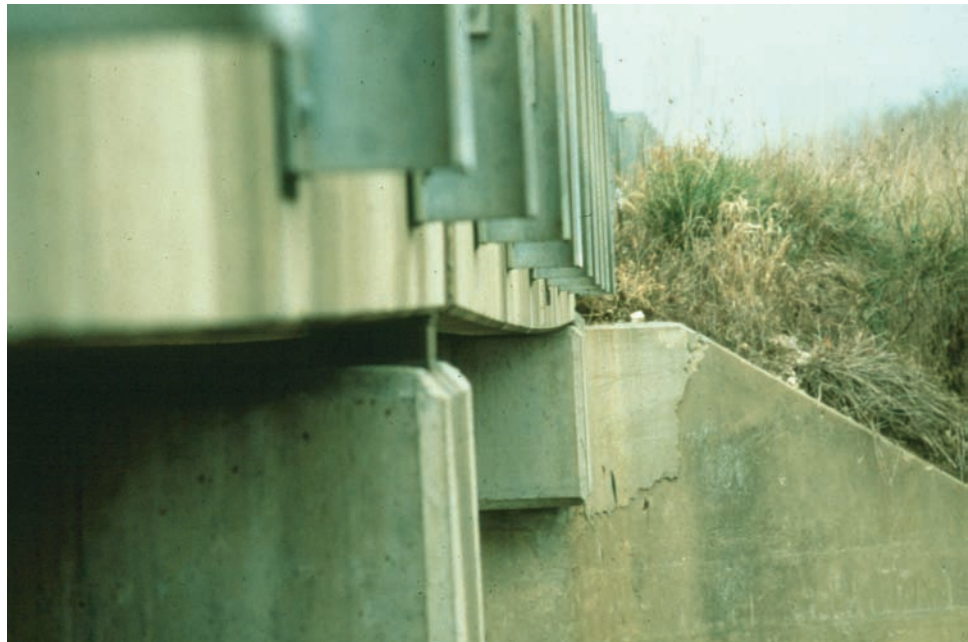
Figure 7.4.5 Excessive Deflection at Midspan
