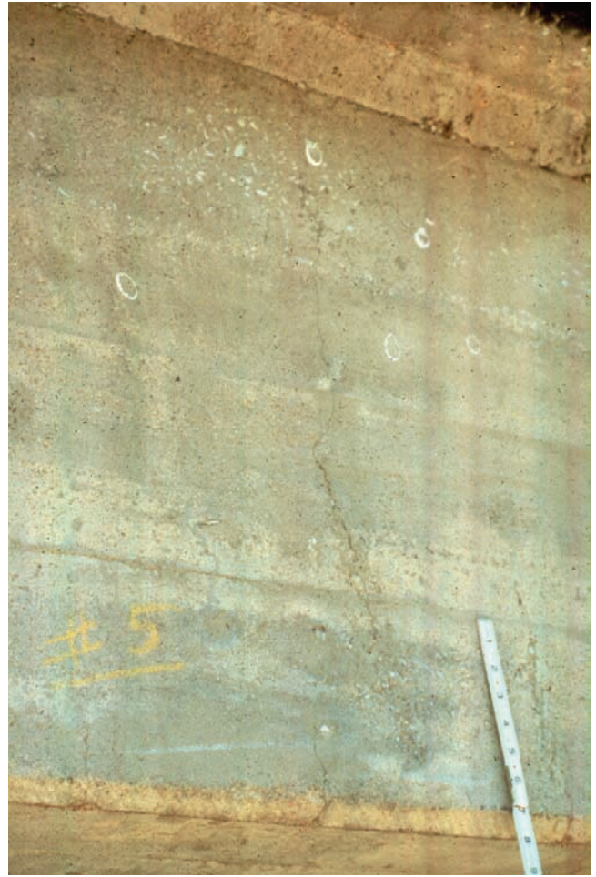
Figure 7.2.13 Flexure Cracks on a Tee Beam
