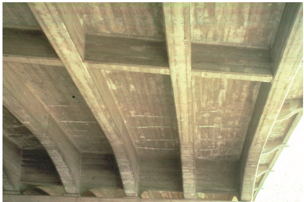
Figure 7.2.14 Flexure Cracks in Tee Beam Deck
