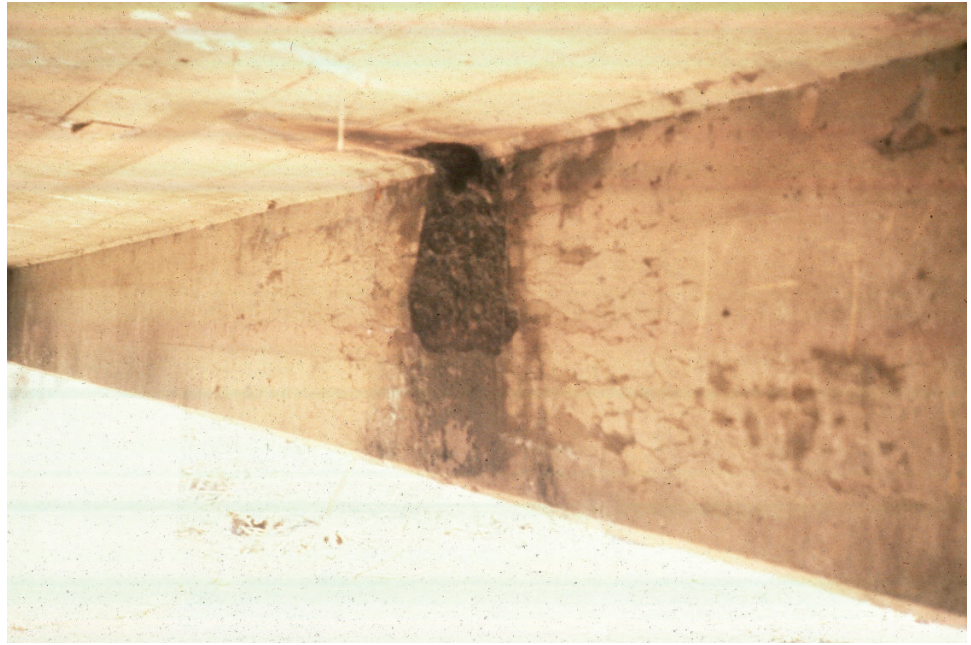
Figure 7.2.18 Deteriorated Tee Beam Stem Adjacent to Drain Hole
