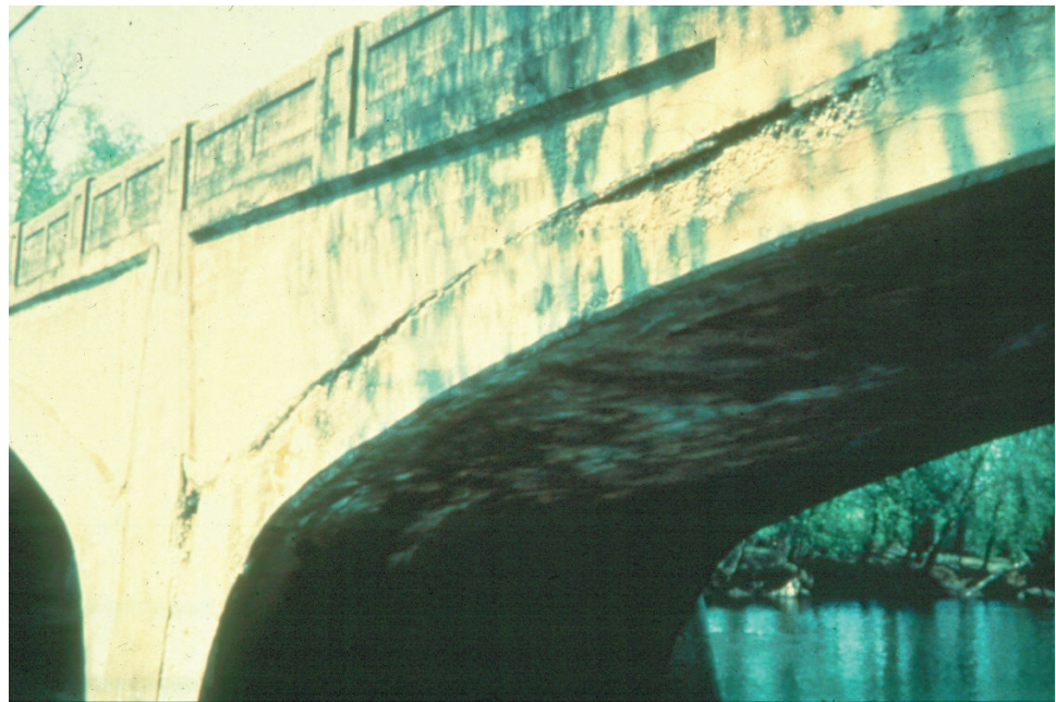
Figure 7.5.16 Deteriorated Arch/Spandrel Wall Interface
