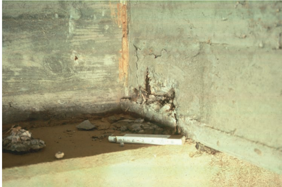
Figure 7.2.10 Deteriorated Tee Beam Bearing Area
